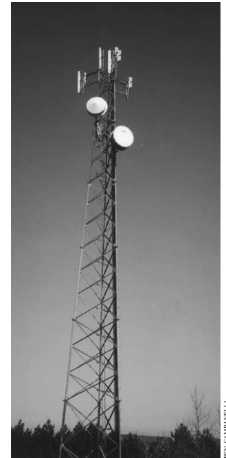
150' Lattice tower with microwave dishes.
