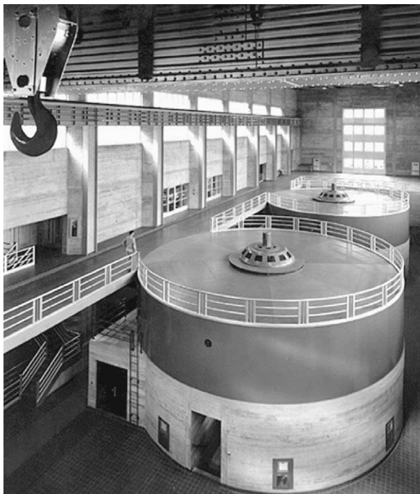
These two huge generators transform the power of falling water into electricity at the Tennessee Valley Authority's Norris Dam.
